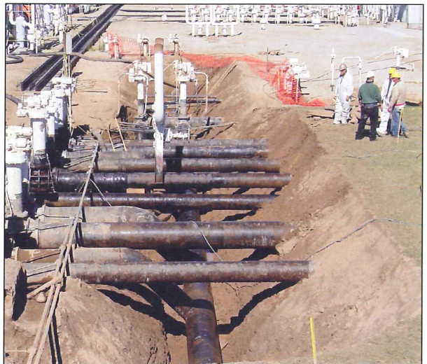
(Left to right) Tom Vilburn, Jim Steiner, Chad Treglowne and Dave McKellar view their recently completed 850-cubic-yard excavation. The hydro-excavation process successfully uncovered and exposed everything underground without disruption or damage.
