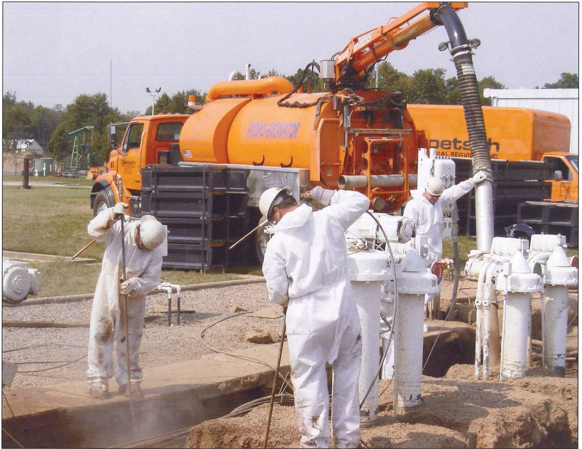
Trenching exposes facilities in preparation for an updated electrical service to a set of control valves.
