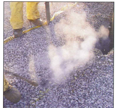
A technician cuts a shallow trench excavation for an electrical conduit run in 15 degree weather.
