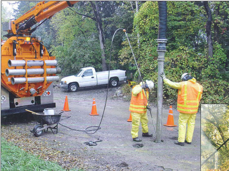
Above, hydroexcavation for a subsurface utility easement. Right, hydroexcavation for a sonotube installation.
