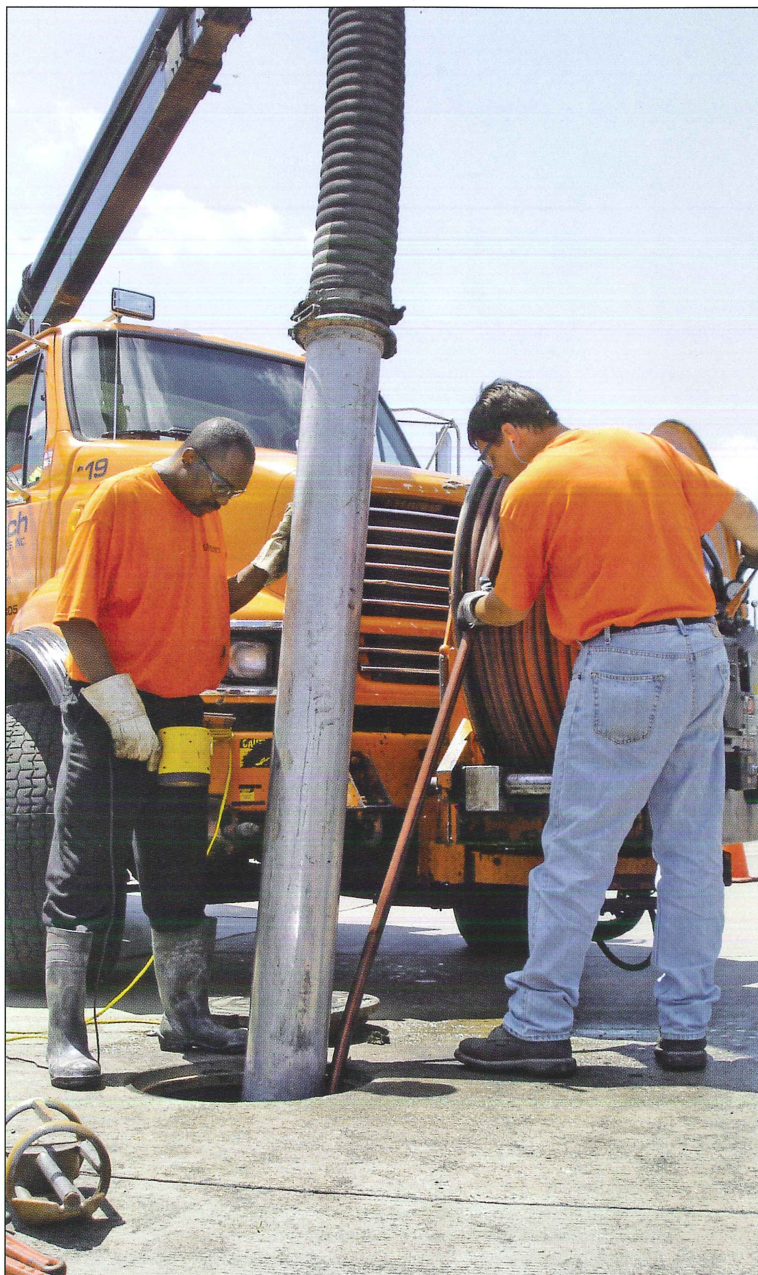
Doetsch Industrial team members use a combination truck to jet a 36-inch sewer line.
