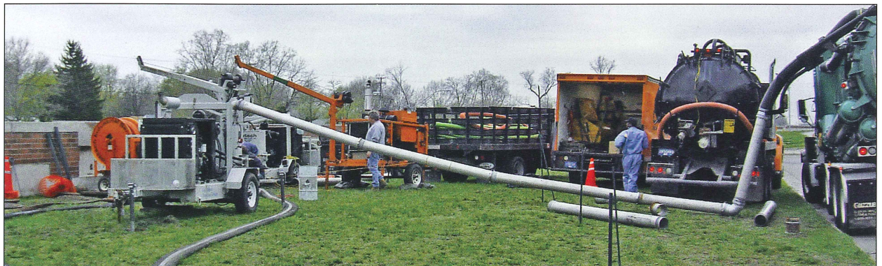
A Doetsch crew and equipment are shown on the site of a siphon pumping and cleaning project.
