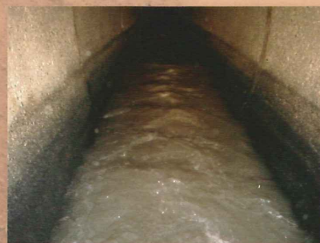
Post cleaning Note: old debris marks
