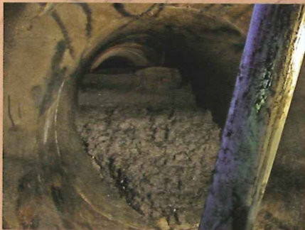
108" pipe with excess debris
